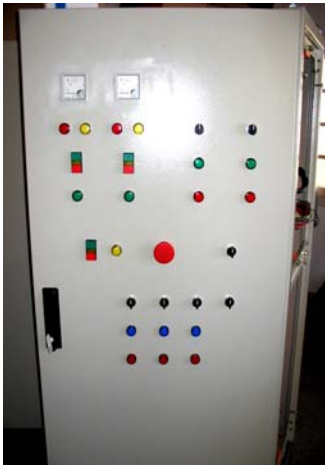
Painel de controle
